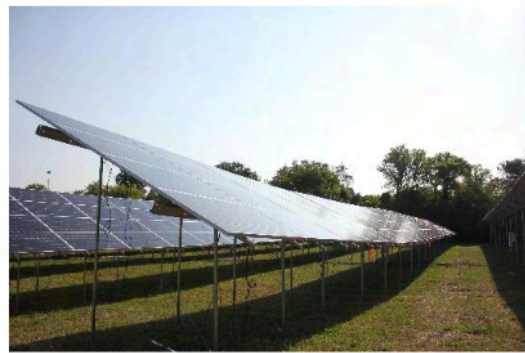
Prairieview School Solar PV System – 634 kWdc
