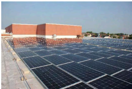
Park Campus Solar PV System – 451 kWdc
