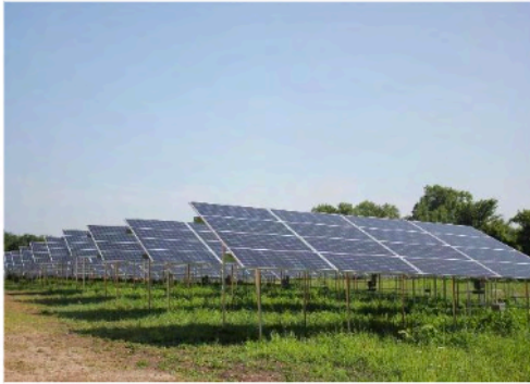
Frederick School Solar PV System – 459 kWdc
